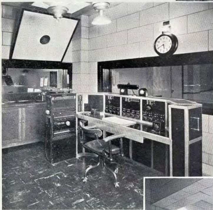
STUDIO MASTER CONTROL ROOM
