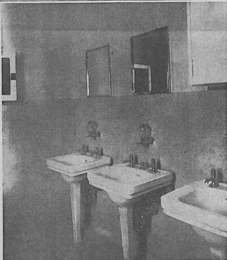
In addition to lavatories and wash rooms on each floor there are also shower rooms. The plumbing and heating work was installed by GRUDEM BROS. CO.
