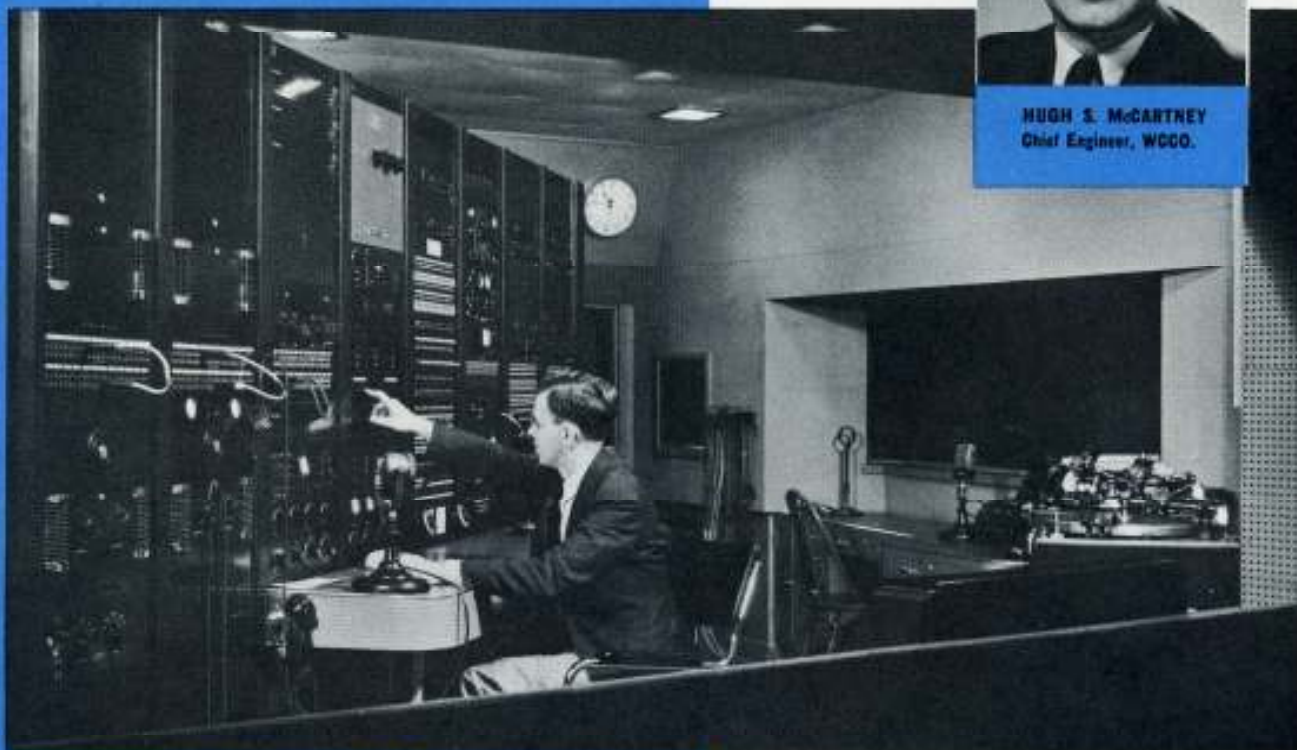
View of Master Control room. Here the technician records music, speech and sound effects into a coordinated whole.
